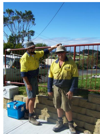
Dan Wright and Jason Smith of Guideline South Coast completing the car park railing.
