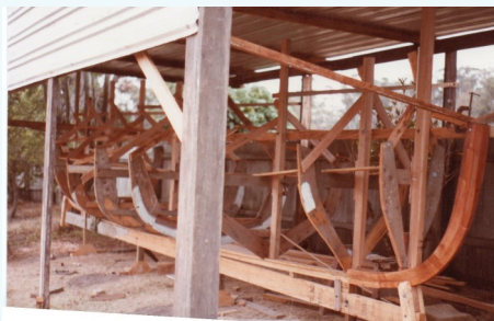
The view over my back fence at the an early stage of Beryl's building
